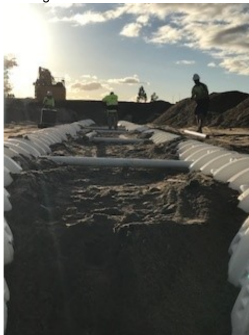
Picture showing balancing pipes
